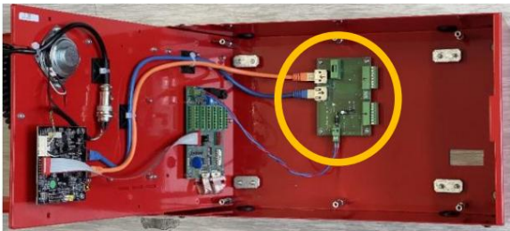
Figure 4: Interior view VAP1-FES
